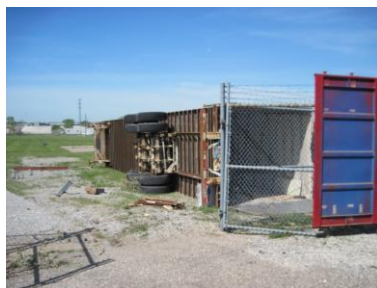
The lumber storage trailer behind the restoration shop was flipped over, and a storage trailer on the ramp was gashed by flying debris.
